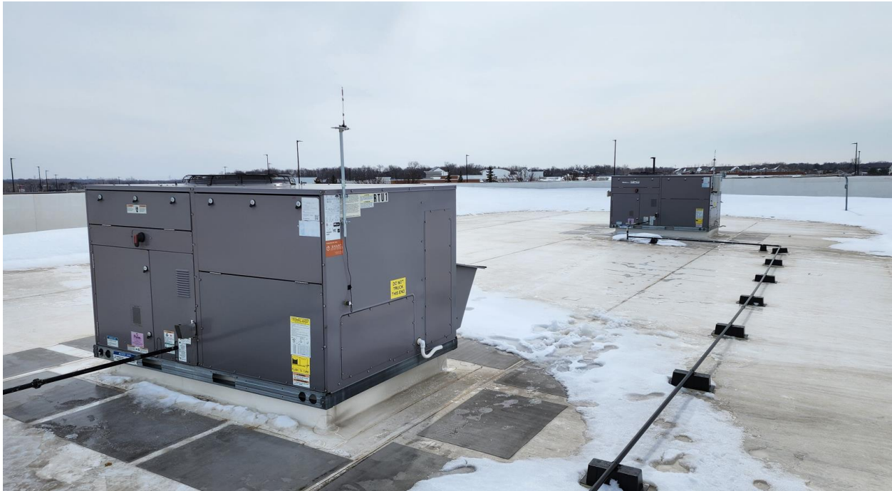
Figure 4. Site-2, RTU-1 and RTU-2
